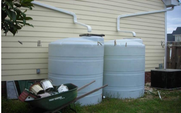
Rain Barrels with Roof Drains
